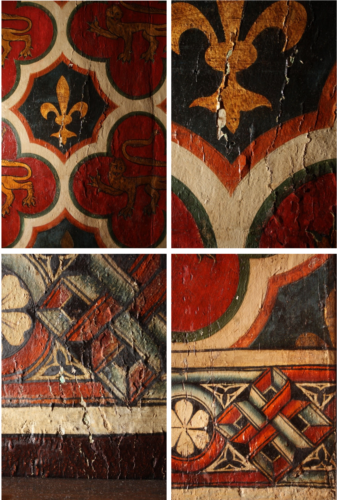
Fig 2. Raking light details of lifting and flaking paint.
